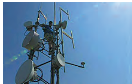
SK7MQ Repeater Tower (Intraframe. Own work. Licenced CC BY-SA).
