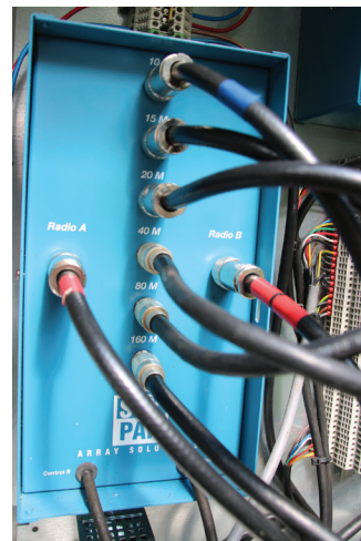
PHOTO 2: Remote antenna relay switch unit housed in an IP65 enclosure.
